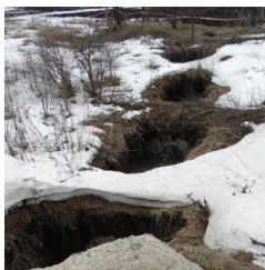
Fig. 1. Sewer deterioration in the area of the Kharkiv Tractor Plant due to biogenic corrosion
