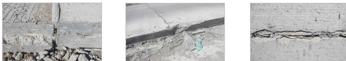
Fig. 11. Contraction joints and expansion joints damaged by slab behavior
