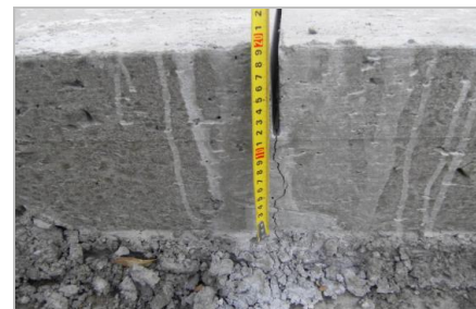
Fig. 9. Form of crack in contraction joints of concrete pavement
