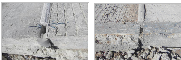
Fig. 10. Measurement of the behavior and length of expansion of horizontally expanded joints
