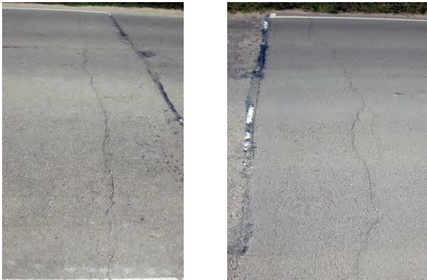
Fig. 5. Thermal cracks on sections № 1 and № 27
