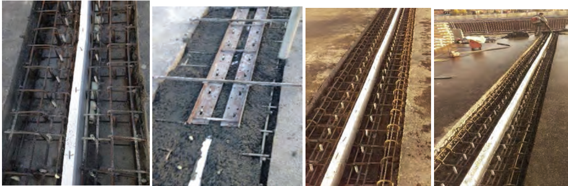
Fig. 9. Expansion joint structure with a rubber compensator with traffic preserved next to it. High-strength concrete was used.
