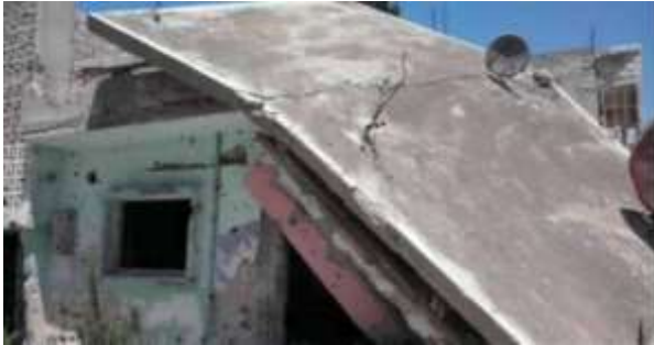
Fig. 8. Partial & total collapse of building
