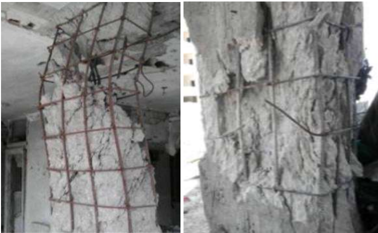
Fig. 6. regular steel reinforcement meshes in column after blast
